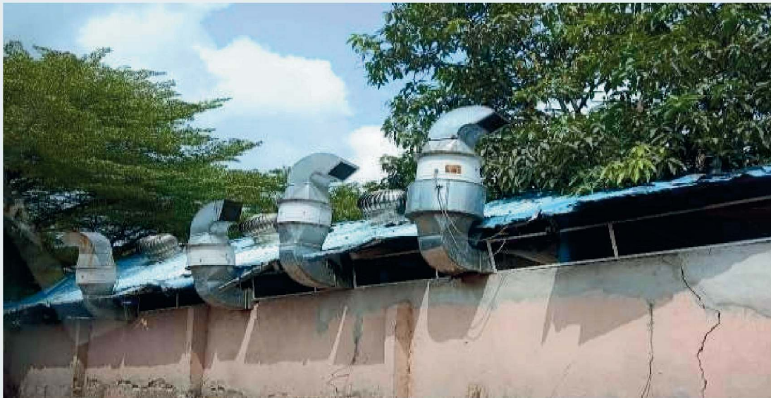
Figure F.5. Outlet of a power plant of a catering company that caters for most of the oil companies in and around Umuseti; their emissions affect the air quality of the environment
