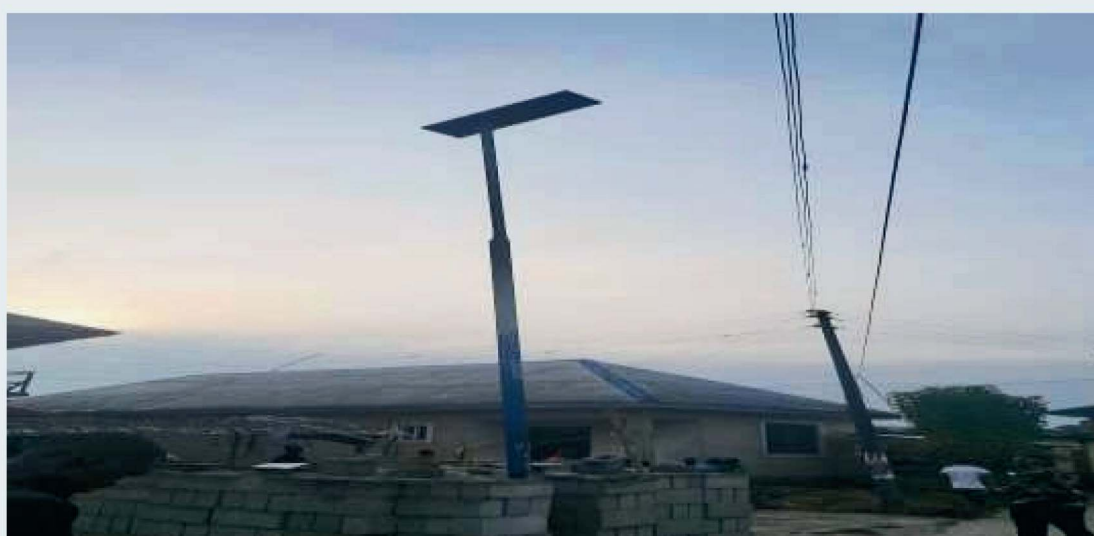
Figure C.5. Solar street light electrification project
