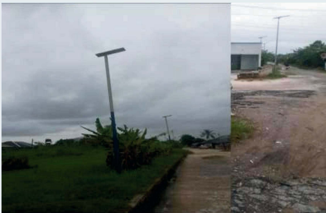
Figure B.2. Solar-powered street lights
