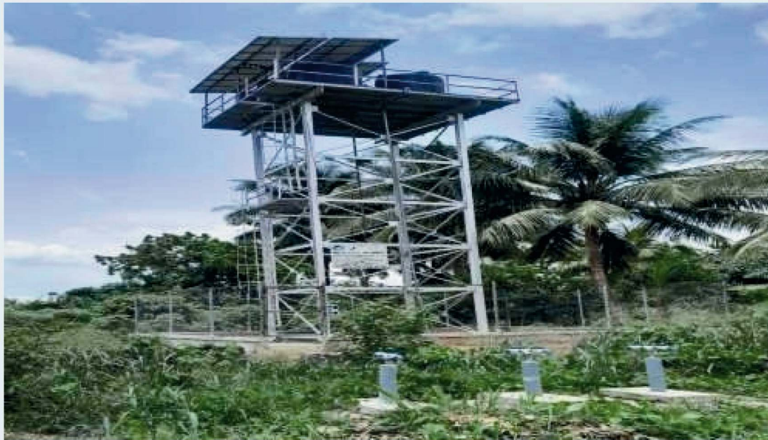
Figure G.3. Solar-powered water reticulation
