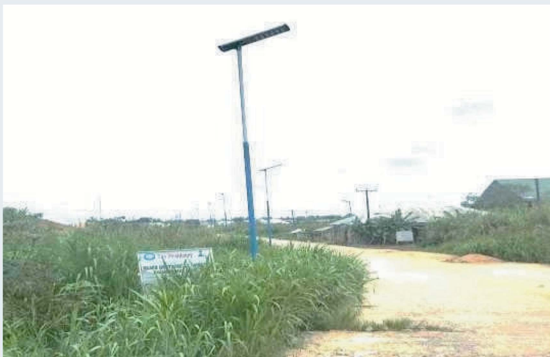
Figure D.3. Solar-powered lights for the streets
